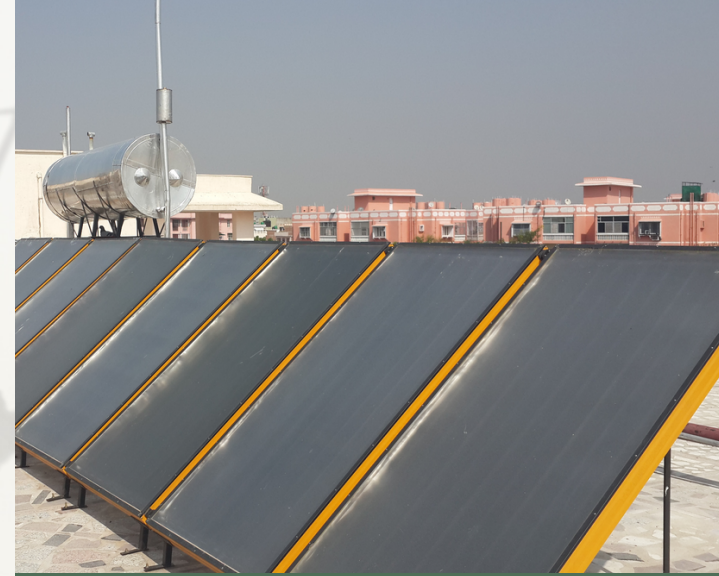
SOLAR WATER HEATING SYSTEMS
